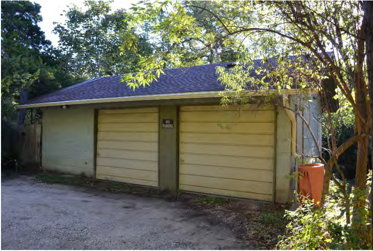
Fig. 4-1-14. Example of a garage located at 3406 Duval Street. Constructed in 1929, this garage is situated at the rear of the main house. It is a one-room wood-frame structure clad in asbestos siding with no stylistic influences. Source: Photo by HHM, 2019.
