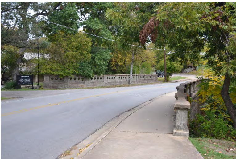
Fig. 4-1-47. This is an example of a transportation resource , Speedway Street Bridge over West Waller Creek, located in Shipe Park. The concrete deck arch bridge was constructed in 1946. Source: Photo by HHM, 2019.
