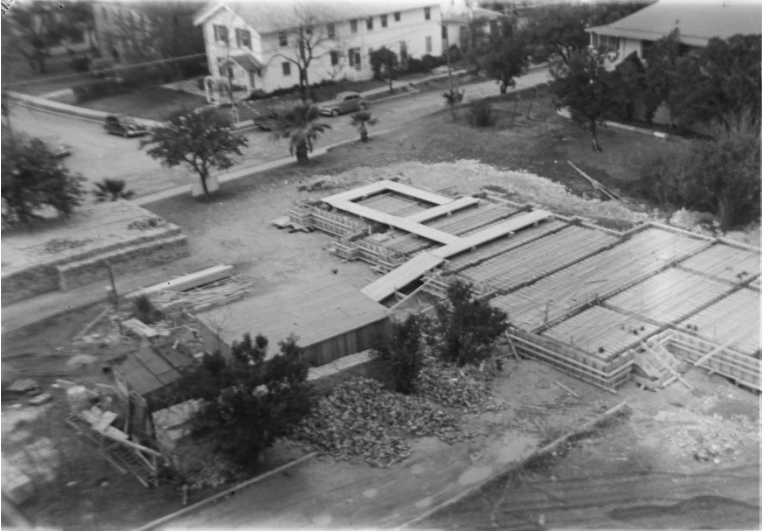
Figure 5-12-4. Historic photograph ca. 1941 of the construction of the Shelton Chapel. One of the seminary's original Mission Revival-style buildings is in the background (hidden by trees in the upper-right corner). Source: The Portal to Texas History .
